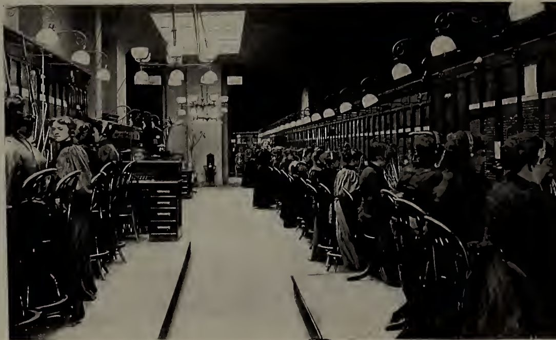
OPERATING ROOM AND SWITCHBOARD, NEW ENGLAND TELEPHONE AND TELEGRAPH CO., 125 Milk Street.
